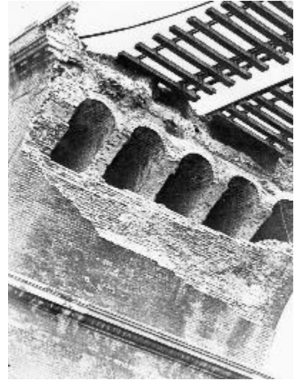
London Road Viaduct after the bombing Brighton and Hove in Picture
